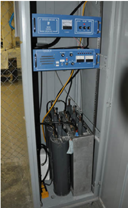
IRARC 146.88 MHz Repeater cabinet at Wuesthoff Hospital. Top unit is the power amplifier, middle unit is the repeater (receiver, transmitter exciter and control board), bottom unit is the repeater duplexer can assembly
