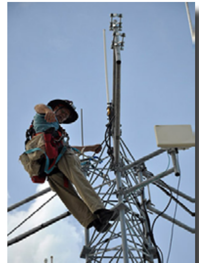
One antenna gone and waiting for the new one. Jim Grossmann, KE4NYN on the harness during the 146.88 MHz antenna replacement
